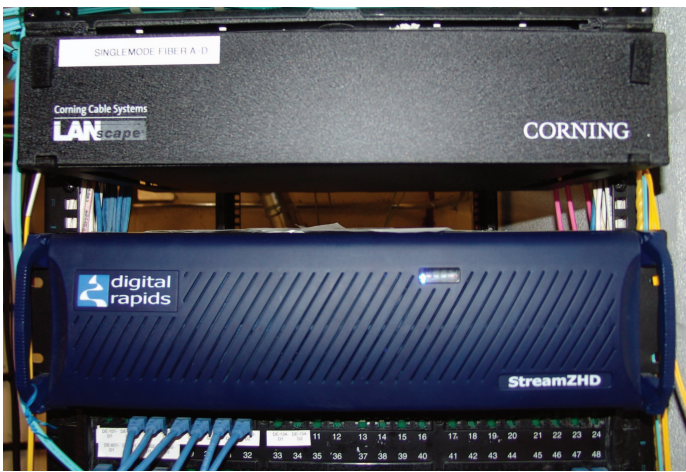
Above: StreamZHD installed in the Lincoln Center data center
